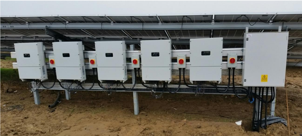
Plate 2-3: Typical string inverter installed under PV modules
