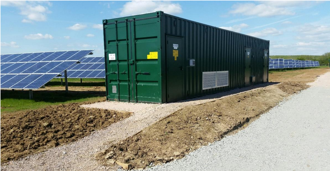
Plate 2-5: Example enclosure containing the transformer and switchgear
