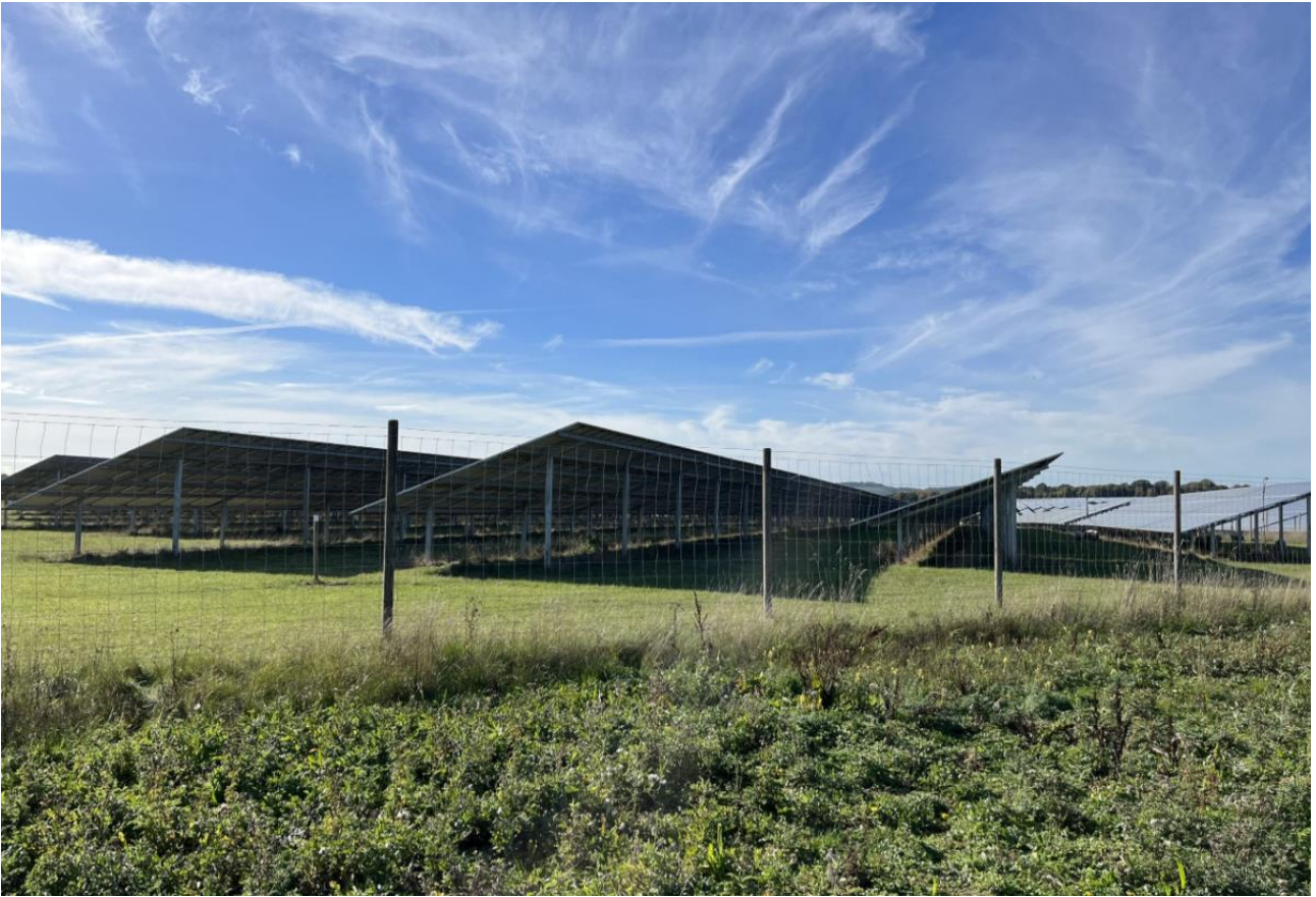
Plate 2-1: South-facing fixed tilt modules, finished array
